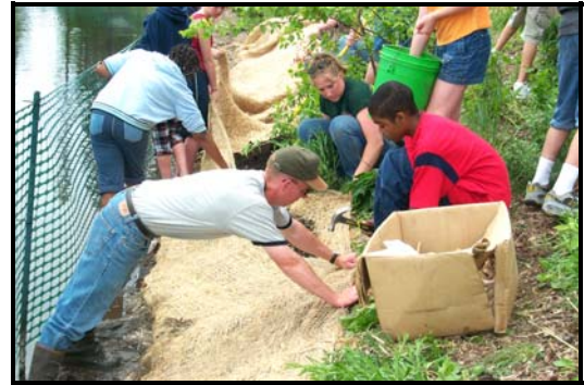
Lee Zabinski, NRCS Technician and students install an erosion blanket and plantings to prevent shoreline erosion.
