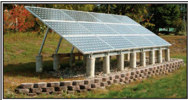
Solar panels at Fairview Office Park.
