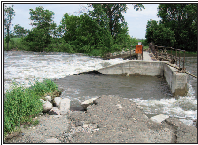
Breckenridge – during its third failure.
