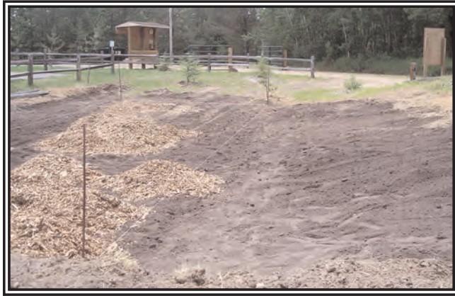
Excavation of the rain garden is complete and mulch is ready to be spread.
